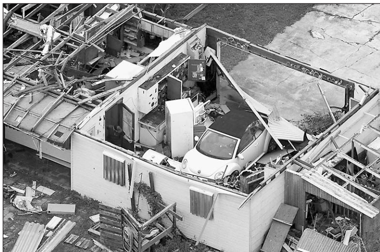
Cars and homes were destroyed by Hurricane Harvey.
