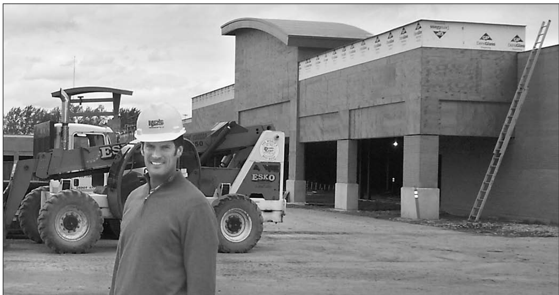
Developer Tom Petzold is in the midst of upgrading the Tech Plaza Shopping Center at 12 Mile and Van Dyke.
